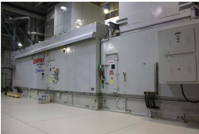
Centrax Trent 60 Generator package
